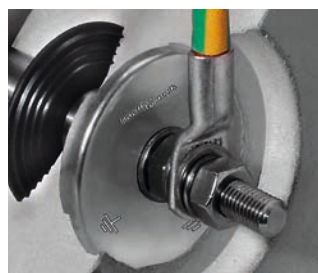
Connected earthing point after removal of the protective cover
