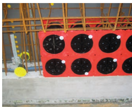
HEA-PK-M12/240 with the PE protective covers fixed at the formwork with nails next to the cable entry HSI 150.
