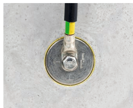
HEA-IS-M12 after the installation. The earthing connection with a cable lug and the contact plate is visible.
