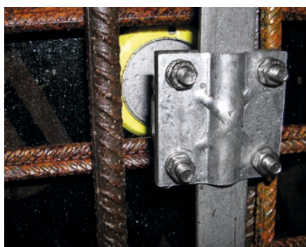
Connection part HEA-P with a screwed-on cross clamp. The HEA-P was fixed at the formwork. A strip steel was included with the cross clamp.
